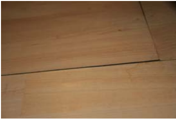
Porous concrete slabs allowing excessive moisture into living areas can cause warping in wood and laminate flooring
