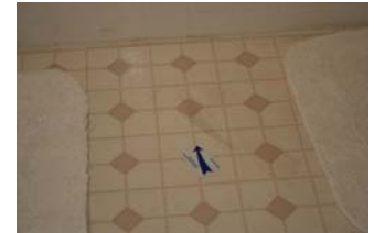
Excessive porosity of concrete slabs can cause deterioration in grout and staining of vinyl flooring
