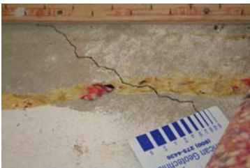
Homeowners are surprised to learn that the concrete slab underneath carpeted, tiled, wood and laminate flooring is often cracked.
