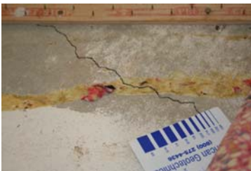
Homeowners are surprised to learn that the concrete slab underneath carpeted, tiled, wood and laminate flooring is often cracked.
