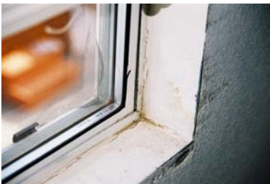
Many window sills are stained, the paint is peeling, adjacent drywall is damaged, and nothing the homeowner does seems to help.
