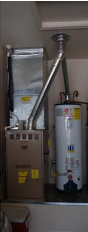
Without exception, every venting system, in every garage that has been examined looks like this – it shouldn’t!
