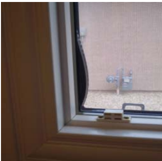
Temperature between the panes increases to the point where the window seals overheat, expand, and lose their shape, causing a loss of the insulation properties of the window.
