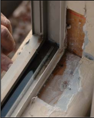
Water intrusion inside your exterior walls results in structural and health issues.
